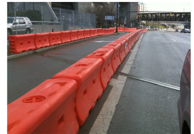
Water-Wall used as a longitudinal channelizer for continuous traffic control delineation for motorists to safely flow through work zone.
